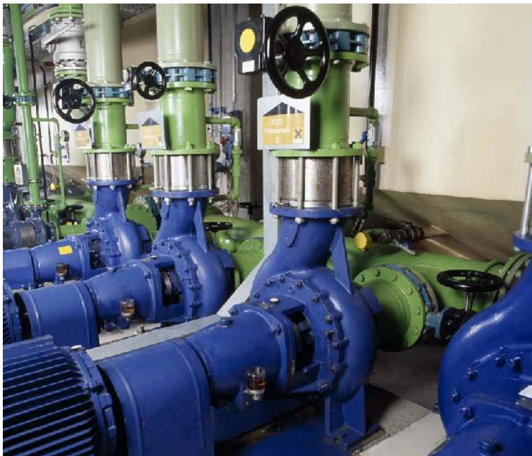
Horizontal motor pump application
